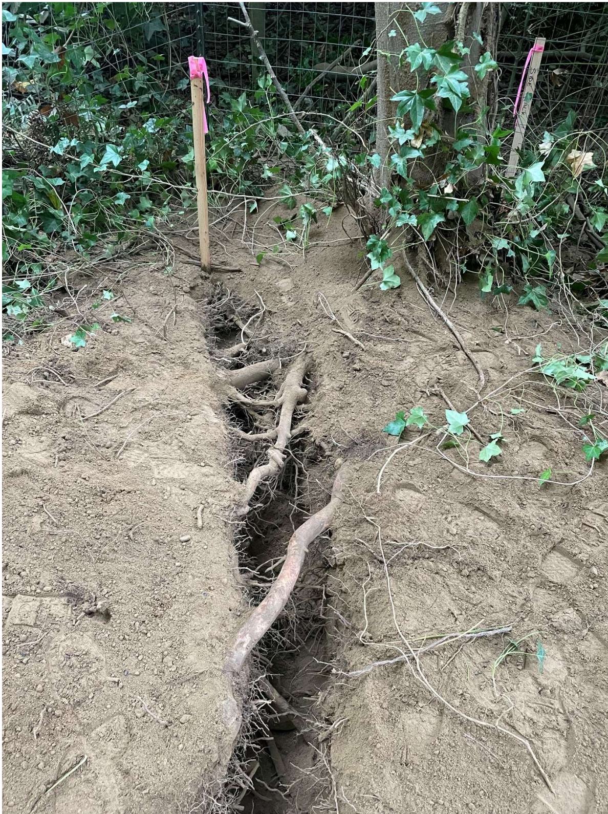
Photo 9. A closeup of the structural roots from tree 1814 found during air excavation of the proposed walkway. None of the roots visible are associated with tree 1813.
