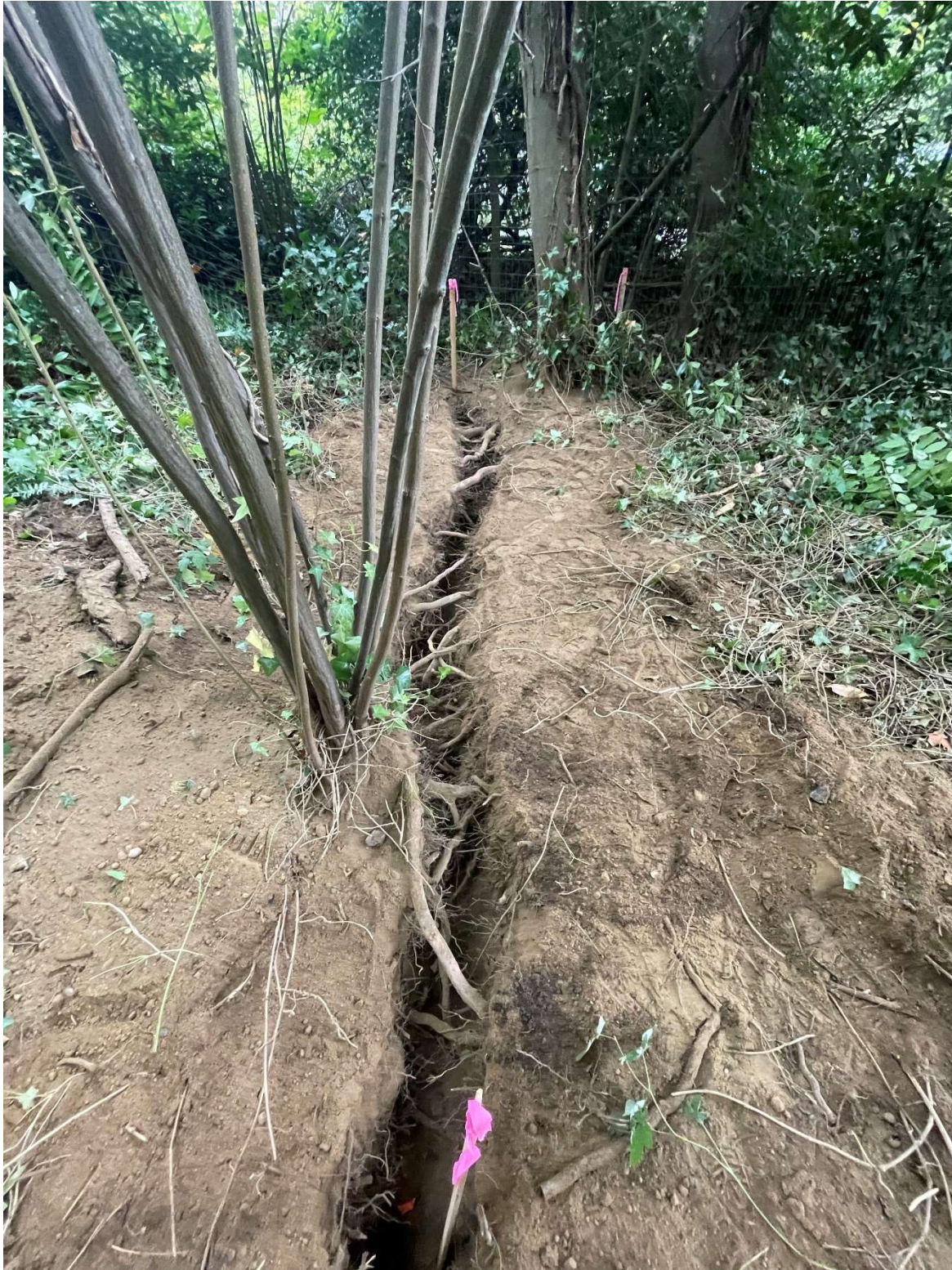
Photo 8. A closer view of roots encountered during air excavation at the edge of the proposed walkway. All visible roots are associated with the non-regulated beaked hazelnut or red alder tree 1814, which is proposed for removal.
