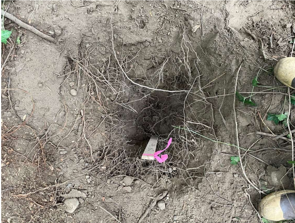
Photo 6. A view of the air excavation at deck footing 1, which is 11 feet to the east of tree 1813. No structural roots were found.
